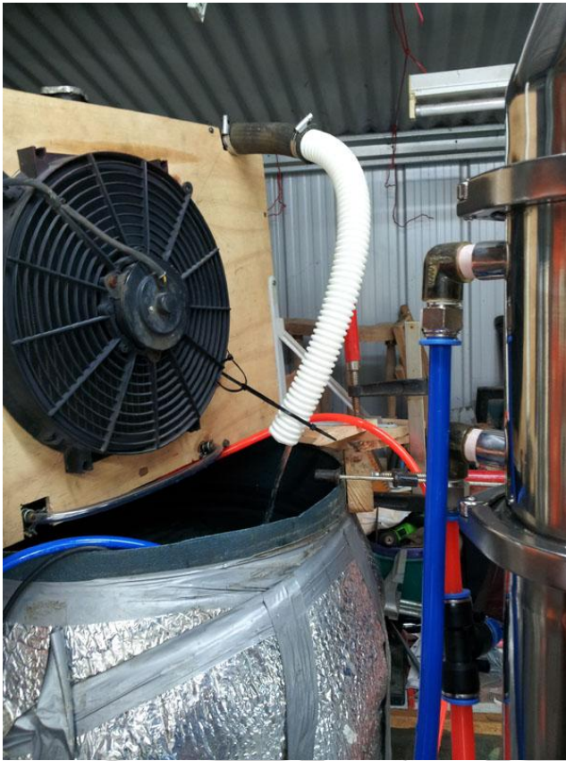
Figure 39: Condenser Connection, Quick Connect Fitting & Thermo Tee
