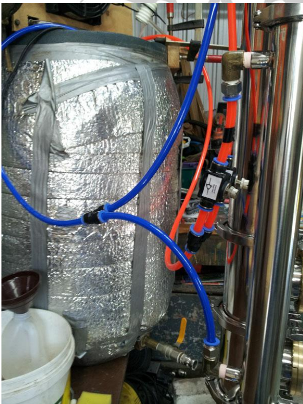
Figure 40: Quick connects, Y Splitters & Needle valves (note direction of flow)
