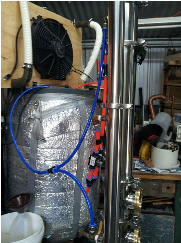
Figure 41: The Authors Plumbing Setup
