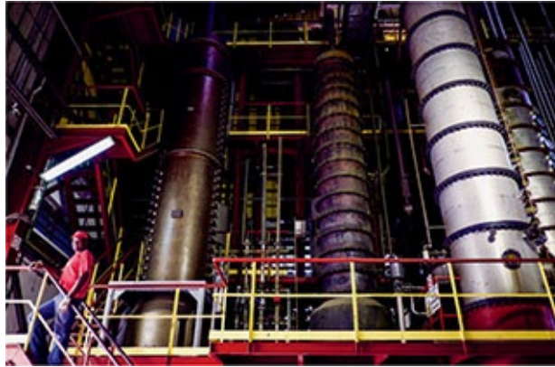
A collection of steel and copper columns of different lengths and widths at the La Mauny distillery in Martinique.
