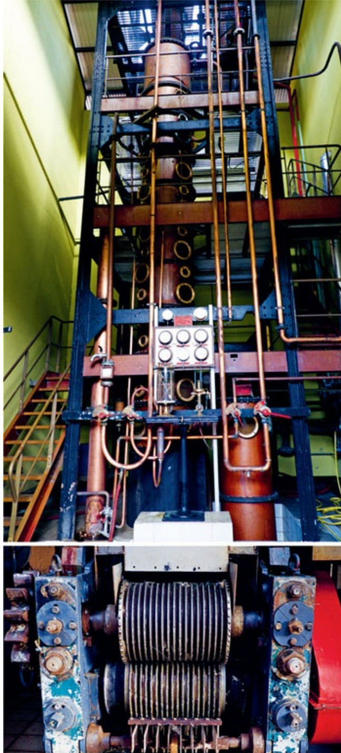
The copper column at Neisson features portholes which make it look like a giant copper octopus tentacle (above); the roller mill at Neisson – it's best not to get too close to these (bottom).
