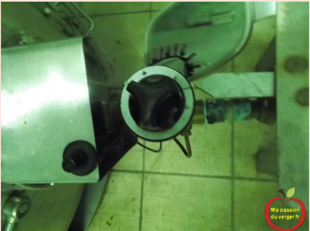
Ignition of the burner.
