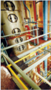
Schenley's huge column stills produce the bulk of the distillery's output.
